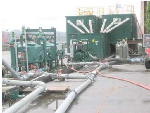
Water treatment system on the Pasley
