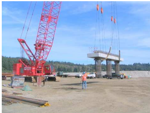
Casting concrete pile caps for the NOAA piers (Photo by Pete Dale)
