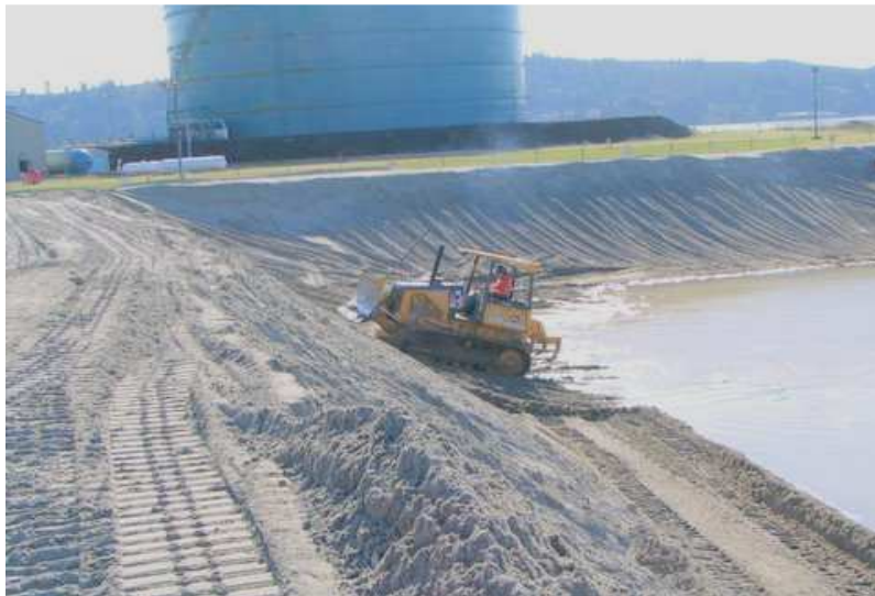
Working on the dredge disposal site near the terminal (Photo by Pete Dale)
